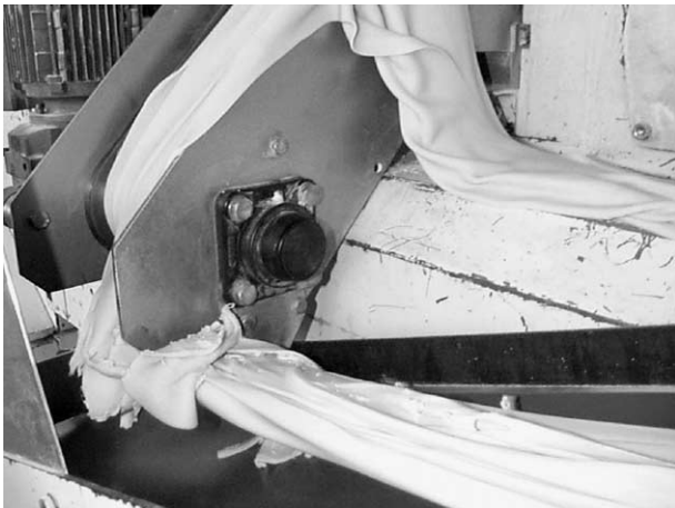
Fig. 4. Bearing as a high risk lubrication point.
